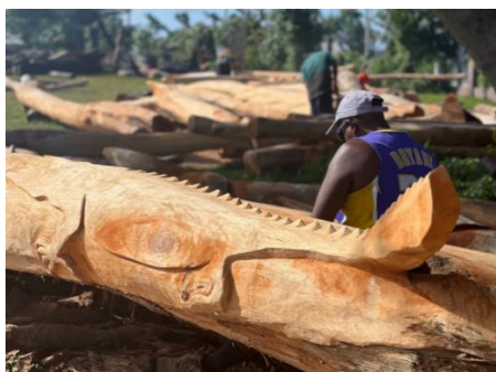
Timber posts being prepared by local carvers to rebuild the Malvatu Mauri Nakamal (meeting house), Vanuatu.
